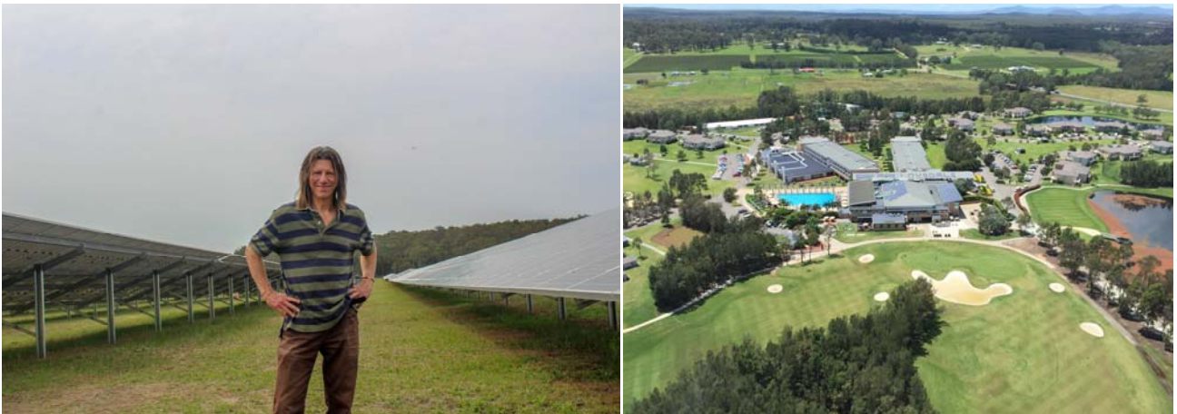
Dr Jerry Schwartz with the new solar installation at the Crowne Plaza Hunter Valley
