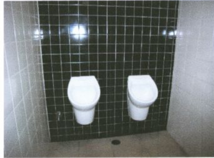
Install Waterless Urinals
