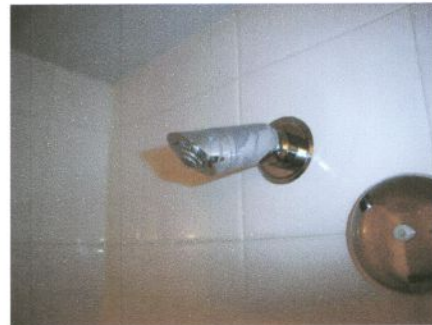
Installed Water Saving Showerheads
