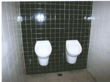
Installed Occupancy Controlled Urinals
